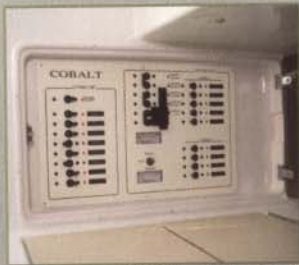
AC/DC Distribution Panel
